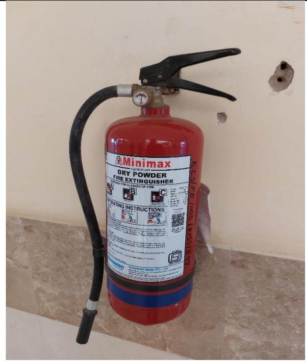
ABC Dry powder type fire extinguisher
