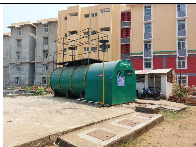
Bio gas plant
